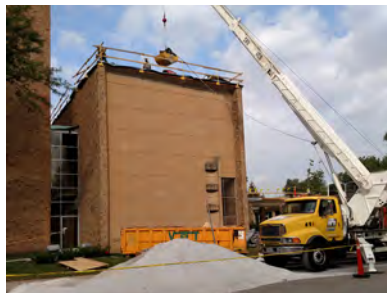
Crane dumping white gravel on the roof for less heat gain during the summer.
